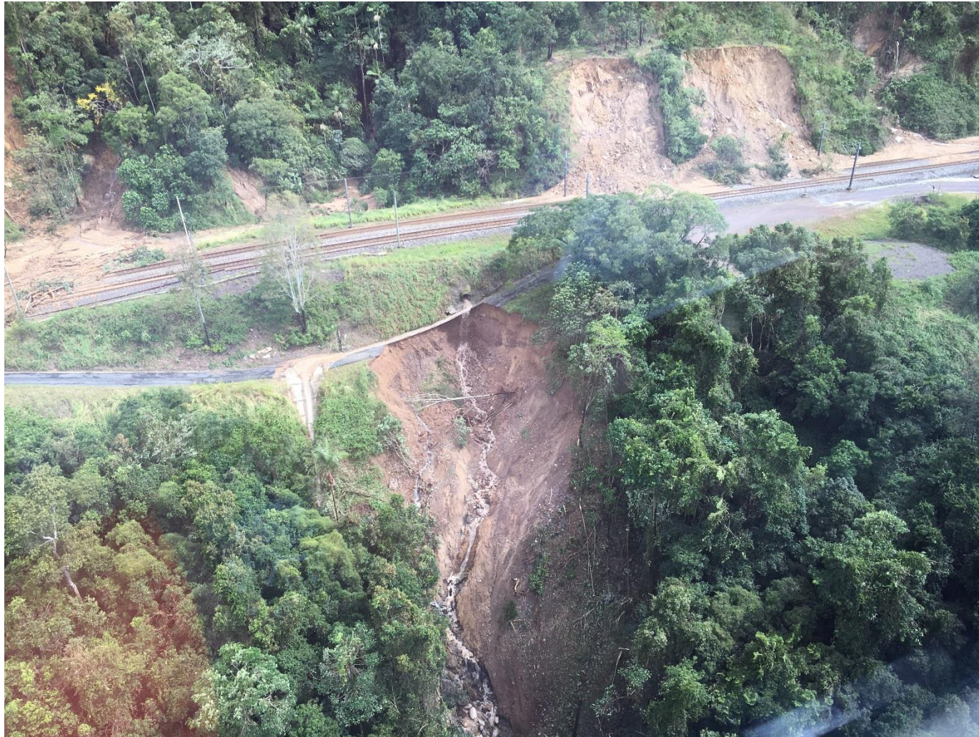
Cyclone Debbie (2017) – Goonyella Chainage GA43.1 km
