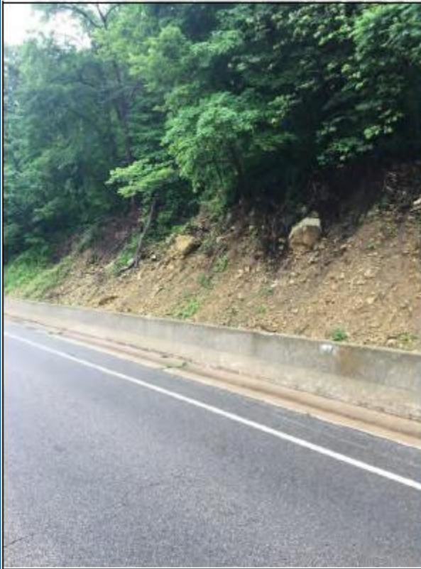
Rockfall sourced from the upper colluvium (typically dislodged boulders that are >1\text{yd}^3 )
