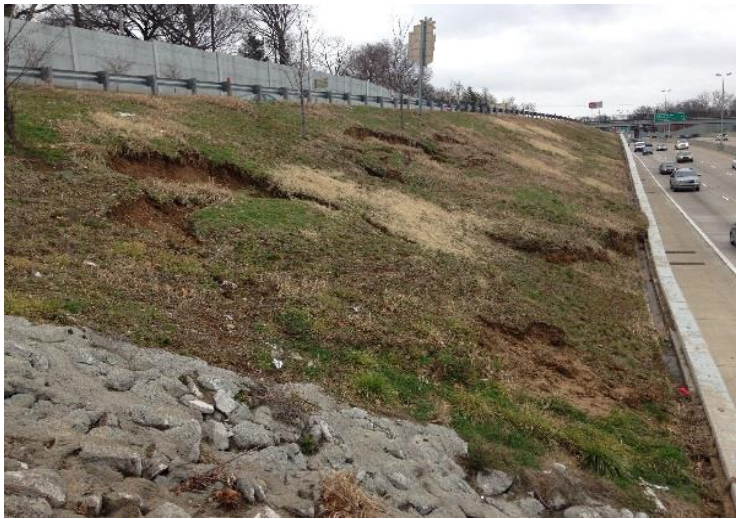
Deteriorating embankment within ROW
